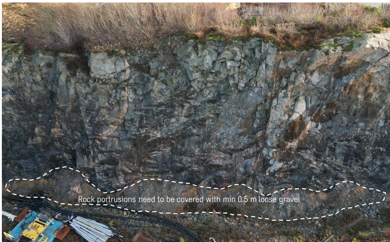
Figure 15 Exposed rock protrusions along the base of the rock cut need to be covered with energy absorbing material e.g. min. 0.5 m of loose gravel.
