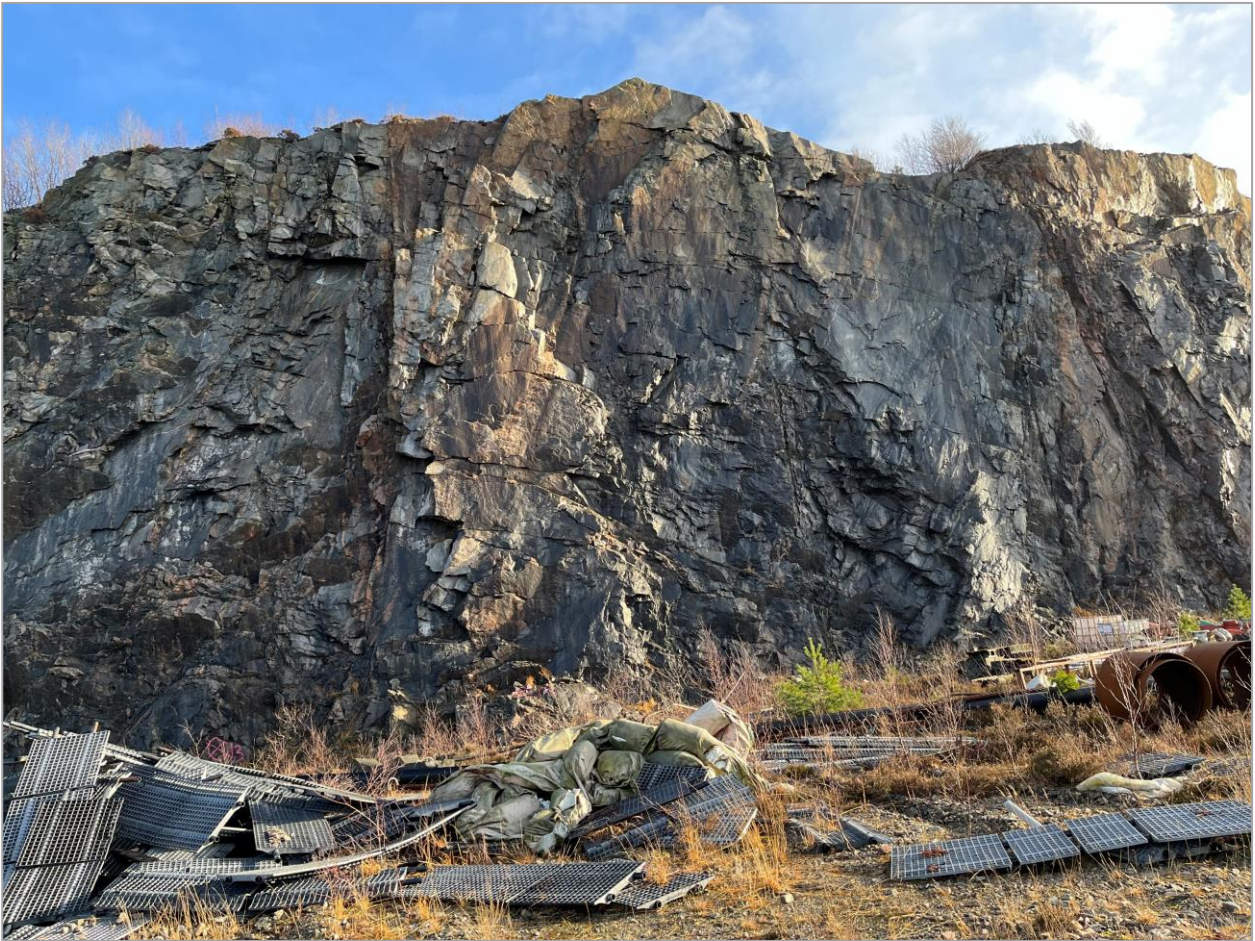
Figure 10 View of a potentially unstable rock column
